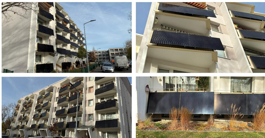
Figure 13: Plug-in PV pilot project in Erfurt, Germany
