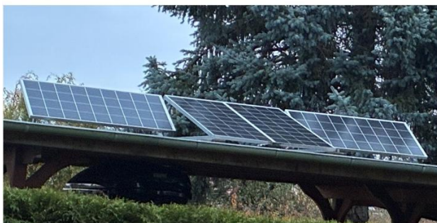
a) Crystalline modules on a carport
