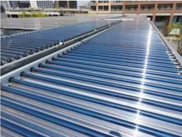
Solar heat panel
