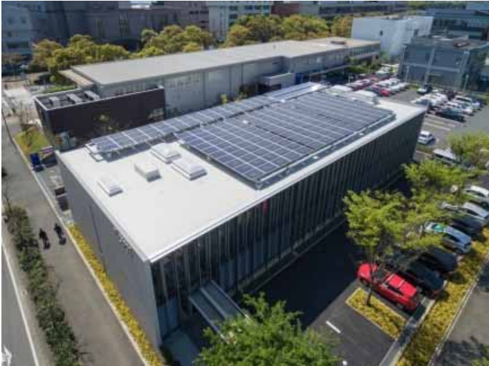
Devices on the roof
