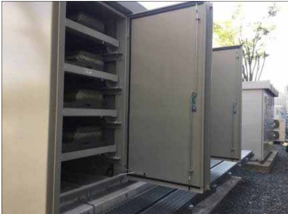
Re-use lithium-ion battery
