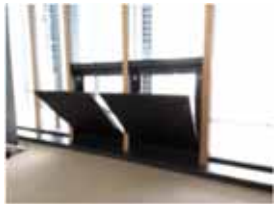
Natural ventilation opening (automatic control)
