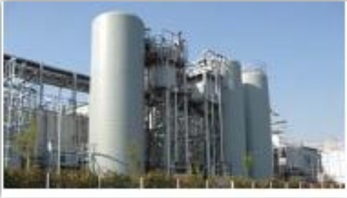
Biogas facility in Kobe Plant
