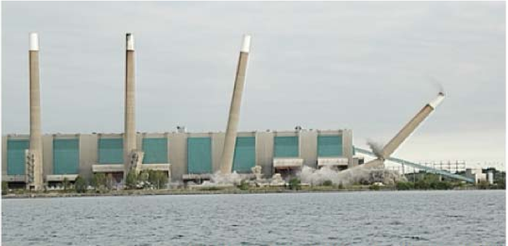
Lakeview Generating Station Mississauga, Ontario June 12, 2006.
