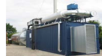
Small CHP- assets
